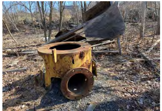
6. View a metal yellow pipe connector on a concrete pad on the northern section of the Site.
