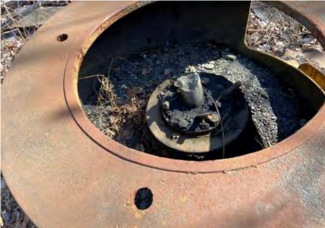
7. View the interior of metal housing.
